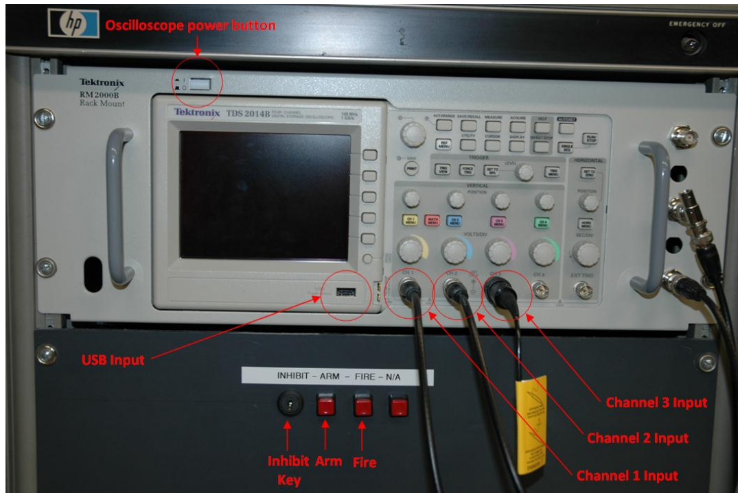
Figure 5.6: Right panel with oscilloscope of the current pulse generator (Hart, 2011)
