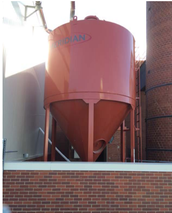
Figure 2.2: Primary Fuel bin
