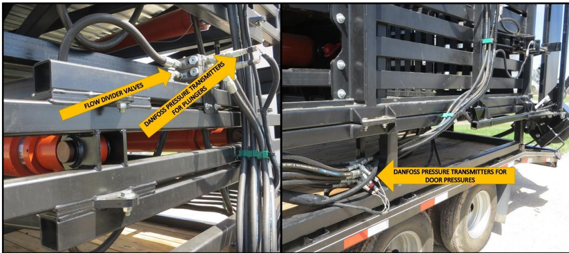
Figure 8.6: Danfoss pressure transmitters used to measure plunger and door pressures
