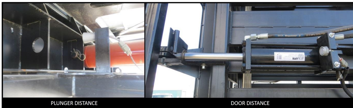
Figure 8.5: Ultrasonic distance sensor used for plunger and door cylinder stroke length measurement
