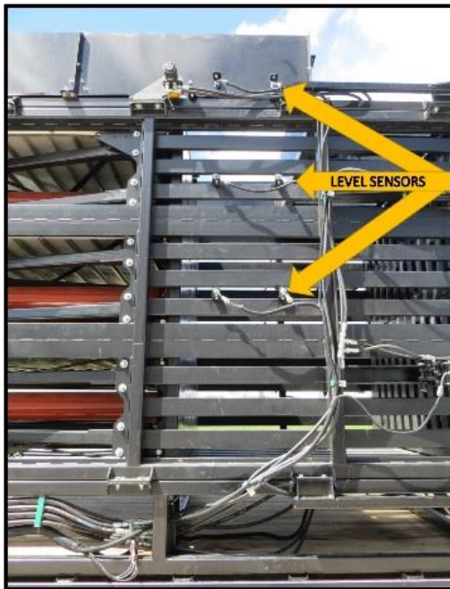
Figure 8.4: Ultrasonic distance sensors used for fill level determination
