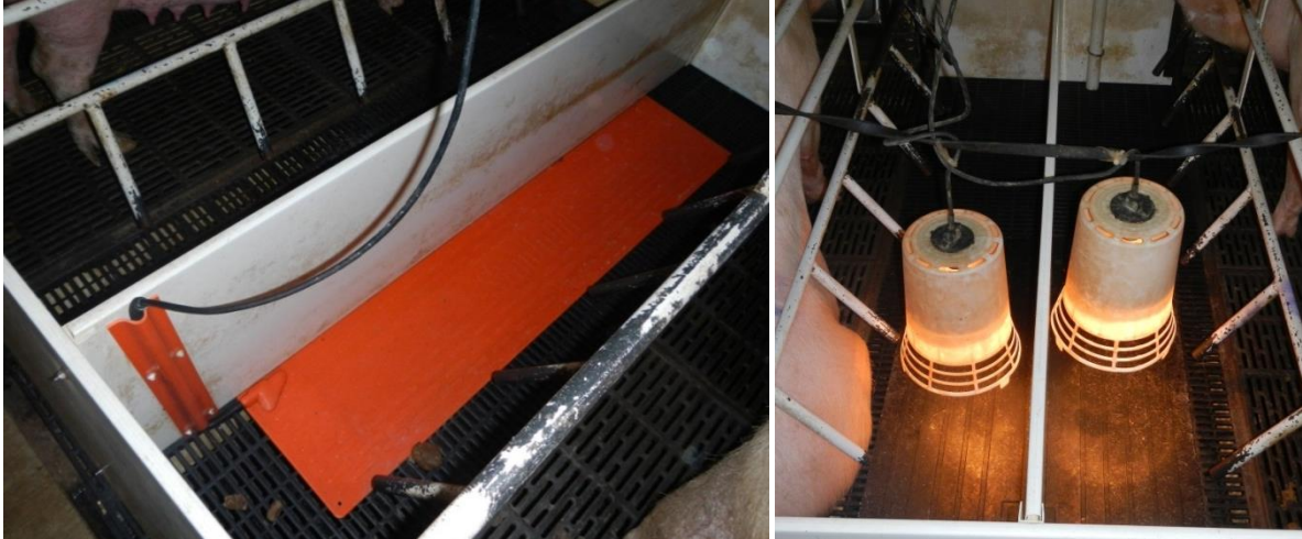
Figure 4.2. Installed localized heating sources in this study: Stanfield double heat mat (0.6 m × 1.5 m) 290W (145 W each side) heat mat (left) and 125 W heat lamps over a 0.6 m × 1.2 m rubber mat (right).
