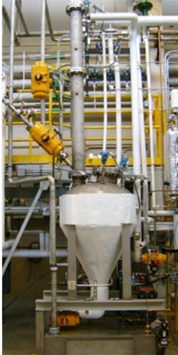
Figure 2: Oil scrubber for tar removal in the PDU
