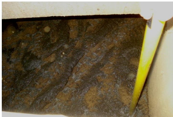
Figure 1. Foam accumulation in a deep pit as seen from a pump-out location.
