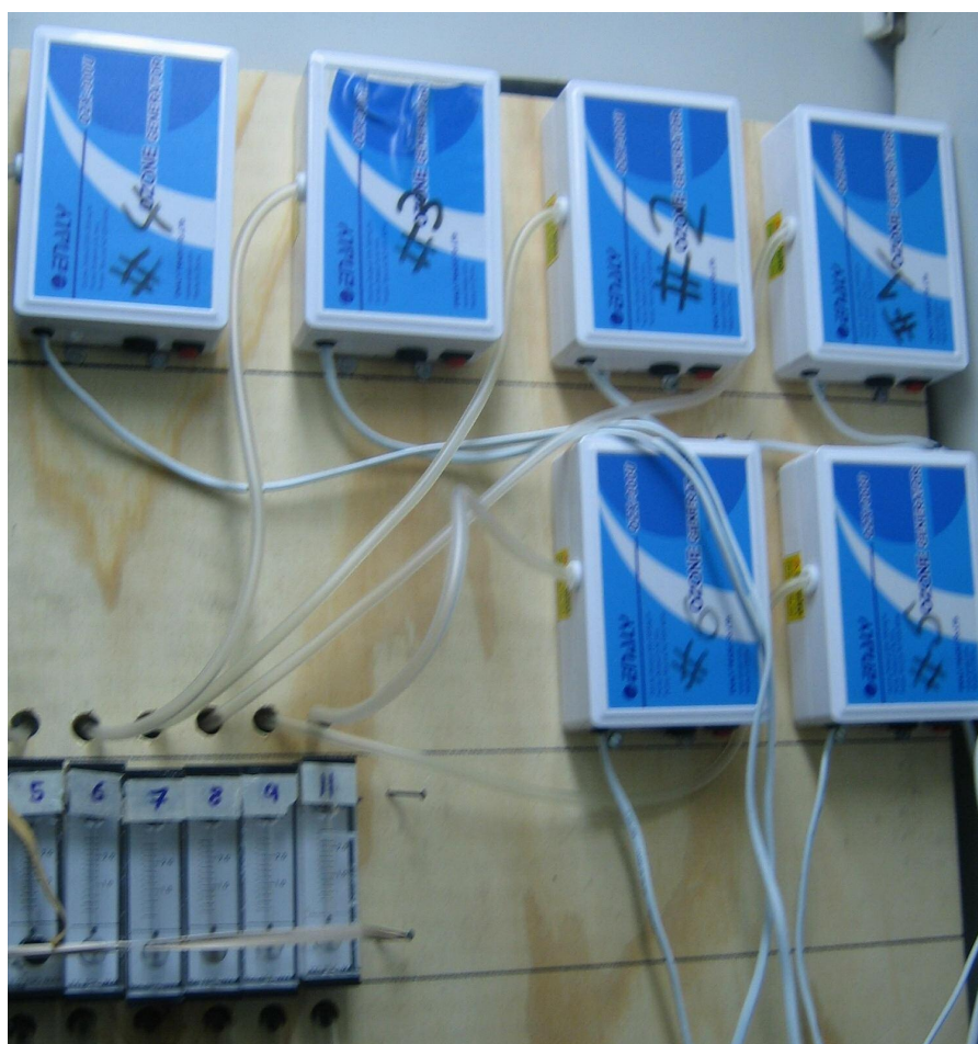
Figure 2.3 Ozone generators and flow meters
