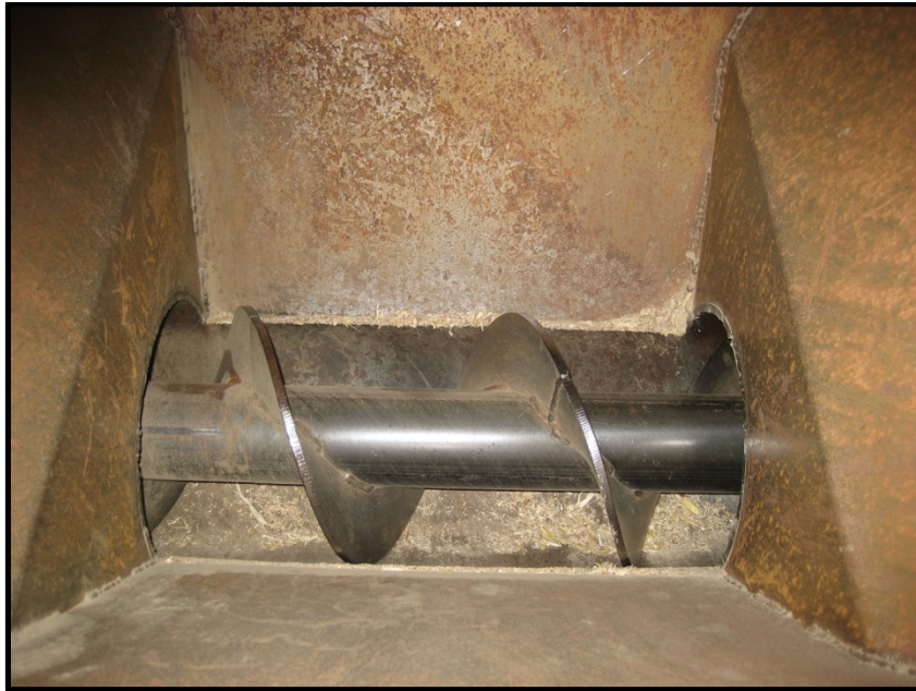
Figure 5. View of the auger from inside the hopper of the auger compaction system.
