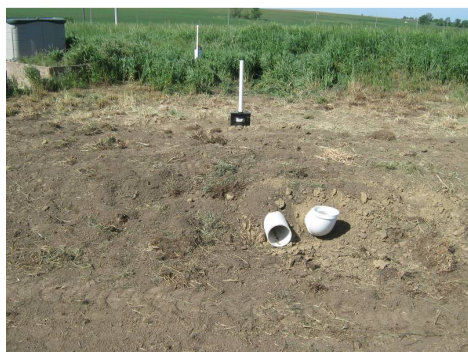
Figure 11a. Northwest IA 1 constructed an earthen berm located in front of the VTA outlet.
