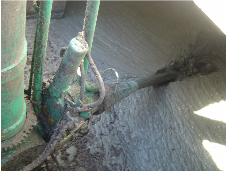
Figure 5.1. A vertical manure pump draws manure and hydrogen sulfide from the bottom layers of the pit and recirculates it into the pit headspace to agitate or mix manure slurry.
