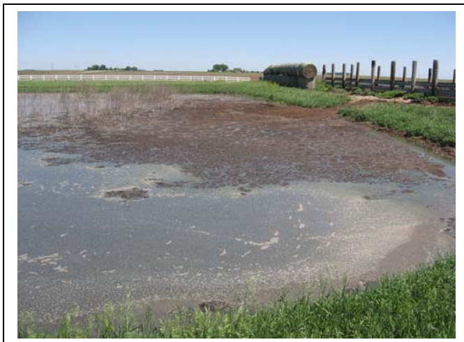
Figure 26: Ponding in the Central IA 2 VIB due to accumulation of solids in 2007
