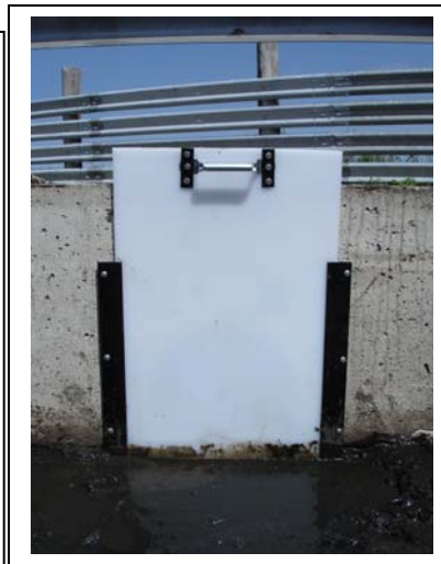
Figure 27: Gate valve installed the Central IA 2 SSB outlet in 2007
