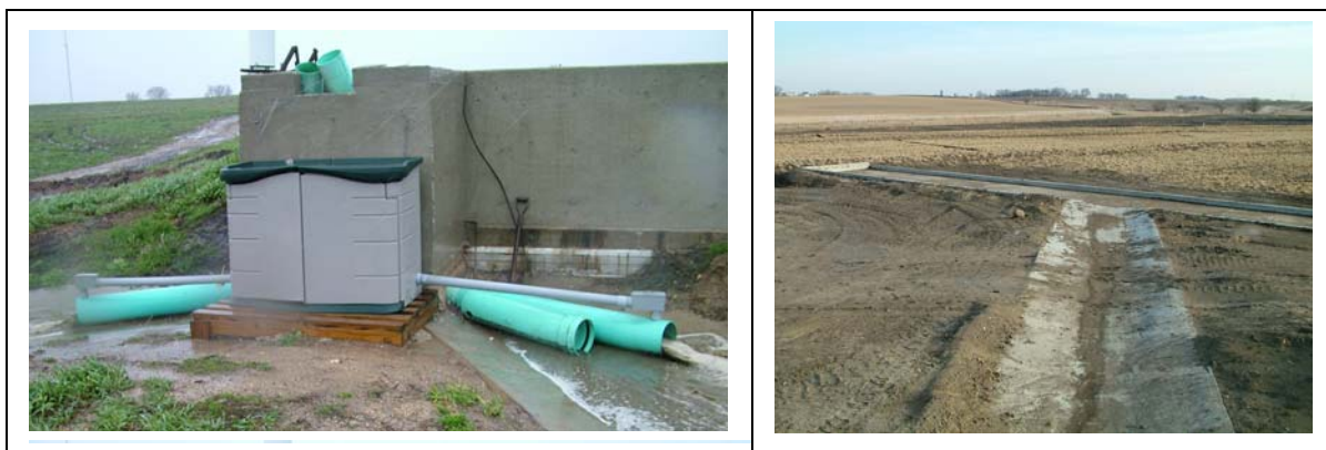
Figure 2: (L to R) Two settling basin outlets; a concrete flow pad leading to concrete flow spreader at Central IA 1
