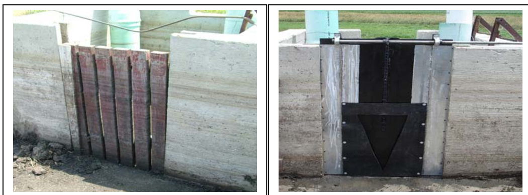
Figure 21: Picket fence at the SSB outlet in 2006 replaced with a gate valve in 2007 at Central IA 1
