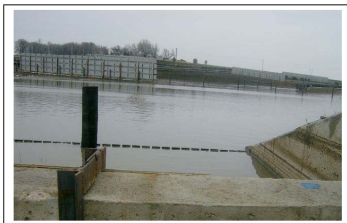
Figure 45: Water backed in the feedlot but the SSB still has several feet of available room
