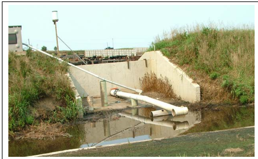
Figure 7: SSB outlet pipe flowing into the concrete level spreader at Northwest IA 1
