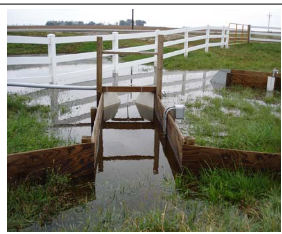
Figure 29: Water backed up in the Central IA 2 VTA flume due to flooding of the roadside ditch
