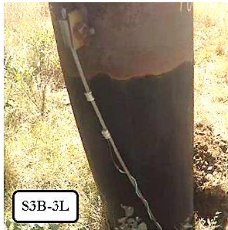
Figure 3.16 Pole S3B-3L showing minor coating delamination but overall dense and adherent patina.
