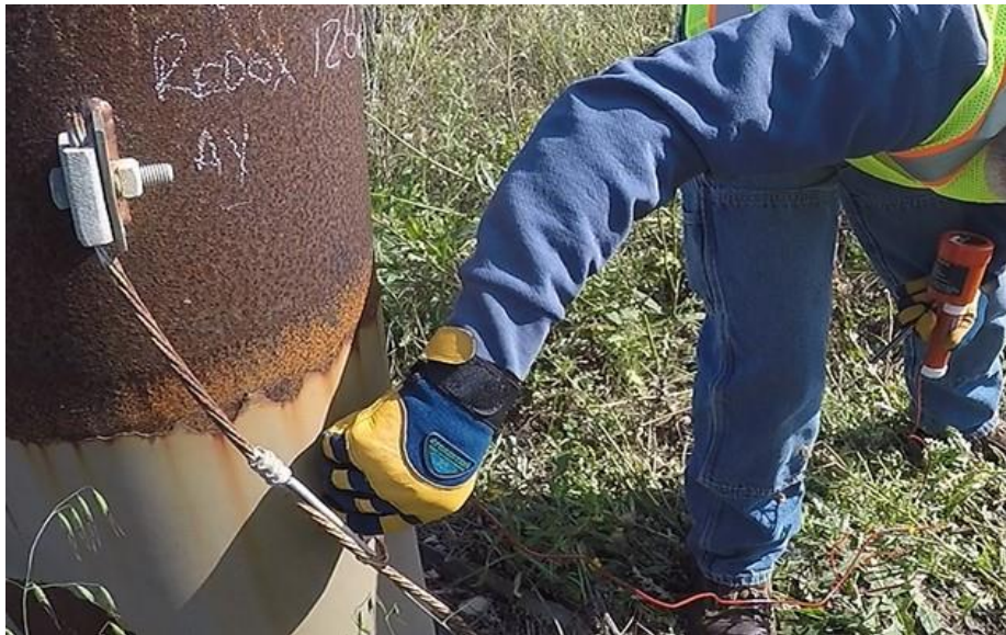
Figure 5.7 Measurement of structure-to-soil potential on WS pole at Site 2.
