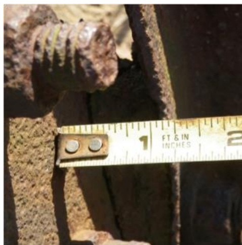
Figure 2.8 Pack-out damage at connection in WS transmission line lattice structure. Note bent steel member.
