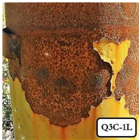
Figure 3.9 Severely delaminated coating line accompanied by widespread pack rust and pack out on ladder clip.
