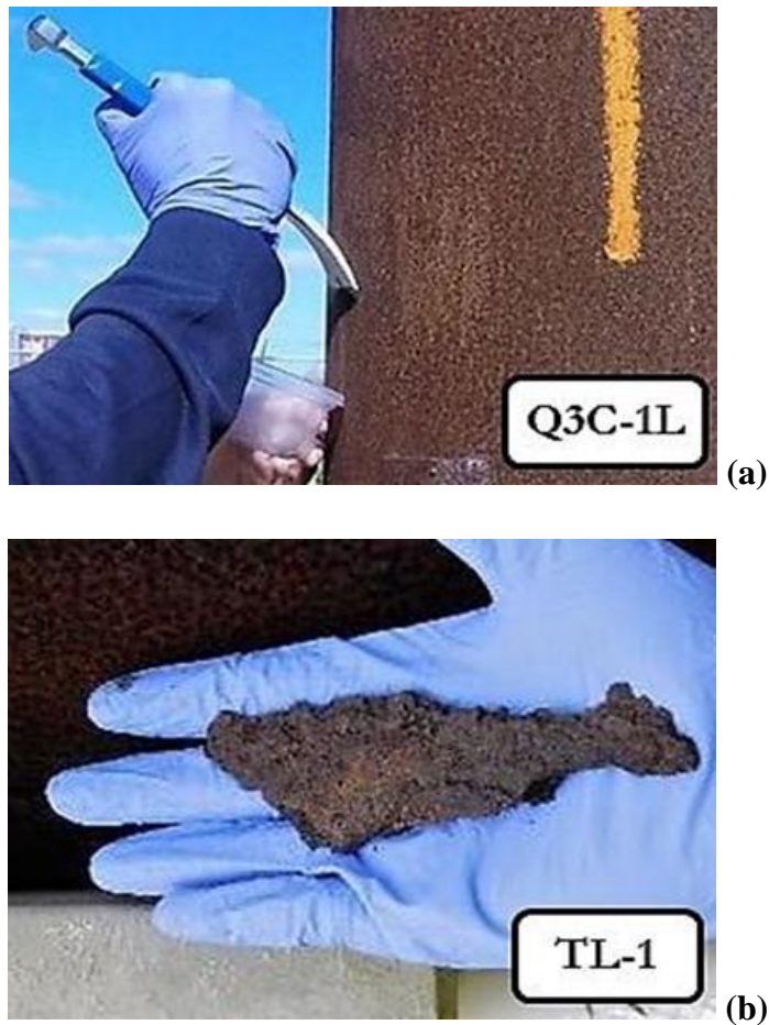
Figure 6.4 Collection of surface oxide samples: (a) scraping of patina to obtain powder sample; and (b) pack-out rust sample removed by hand from junction box area of Pole TL-1.
