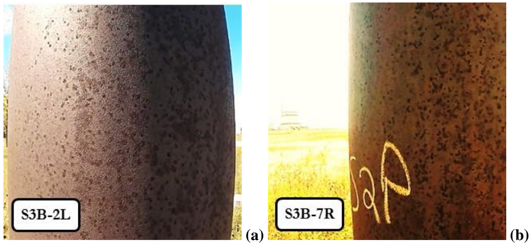
Figure 3.15 Dense pitting sites on pole wall surfaces: (a) Pole S3B-2L facing power station; and (b) Pole S3B-7R facing coal company.
