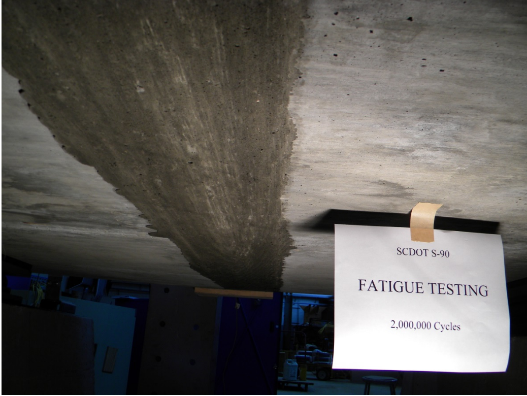
Figure 3.23: Underside of joint after fatigue loading
