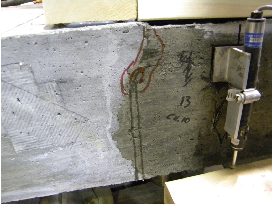
Figure 3.25: Leaking at end of joint
