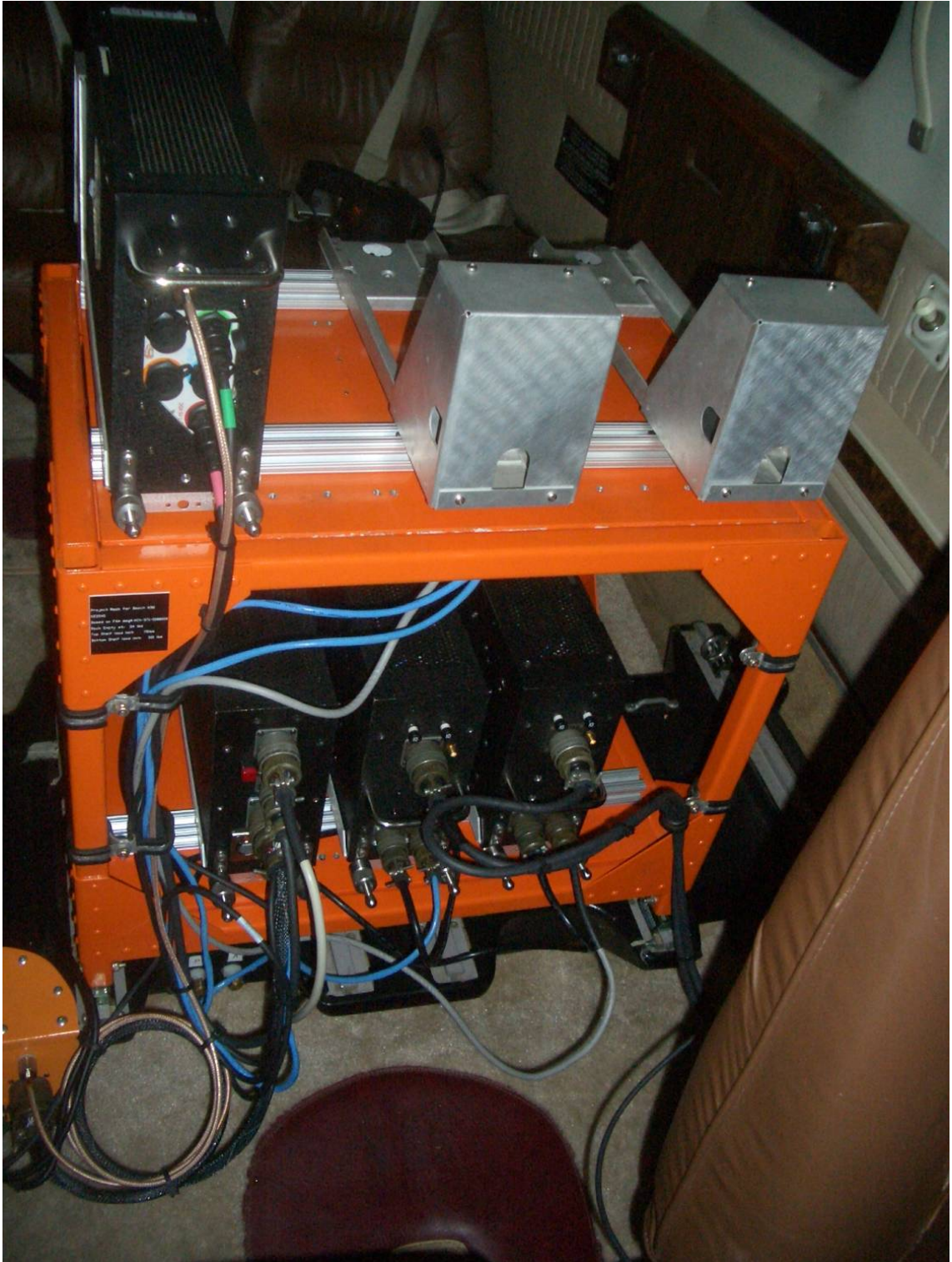
Figure 62 Equipment rack as installed on the middle-row seat rails.
