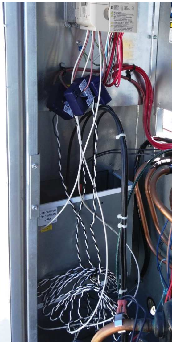
Figure 2.8 Installed CTs on RTU-1 at Muscatine Armed Forces Reserve Center.
