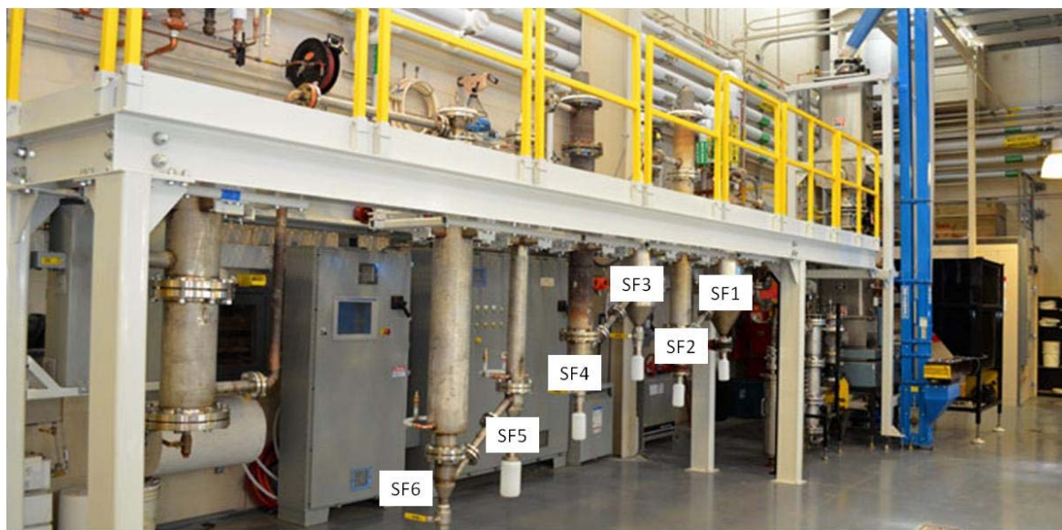
Figure 3 Iowa State University Bubbling Fluidized Bed Pyrolysis Process Development Unit
