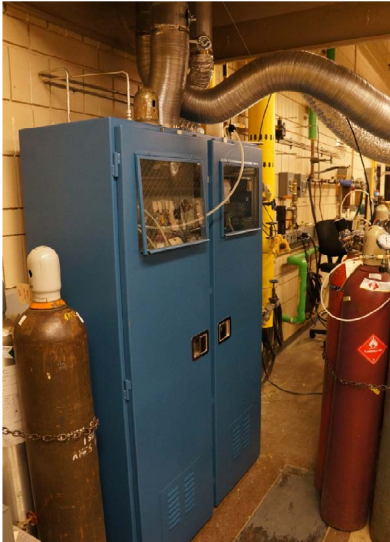
Figure 4.4 vented gas supply
