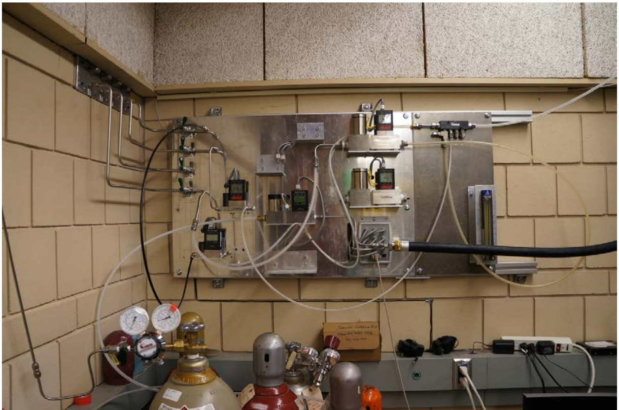
Figure 4.3 Mass flow controller setup
