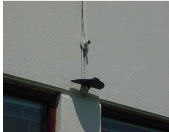
Figure 5: Exterior Lighting Sensors
