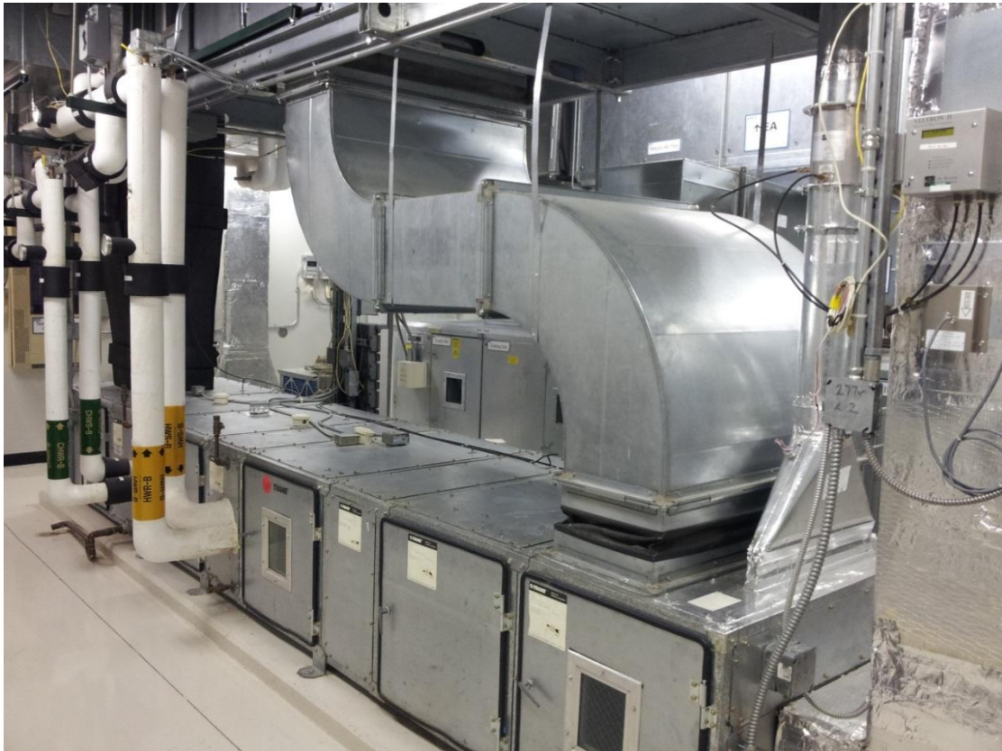
Figure 15: ERS Test Room Air Handling Unit B (AHU-B)
