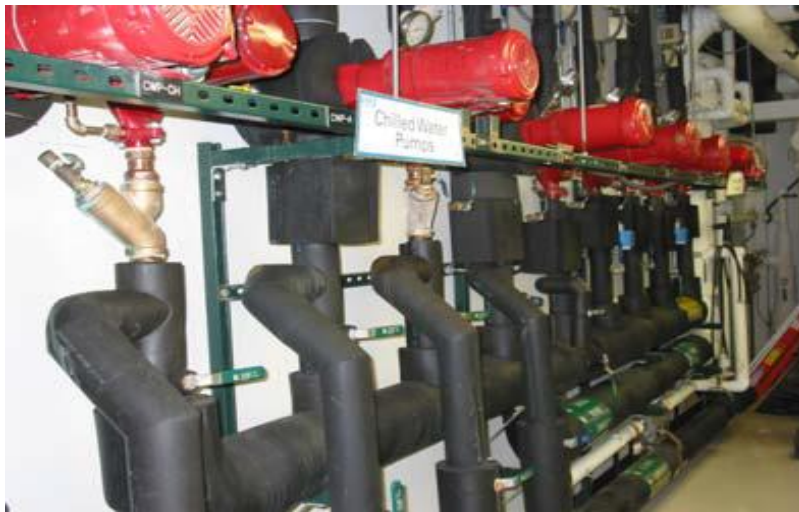
Figure 12: Chilled Water Pumps
