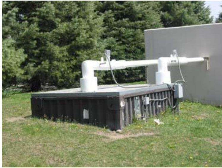
Figure 11: Thermal Storage Tank
