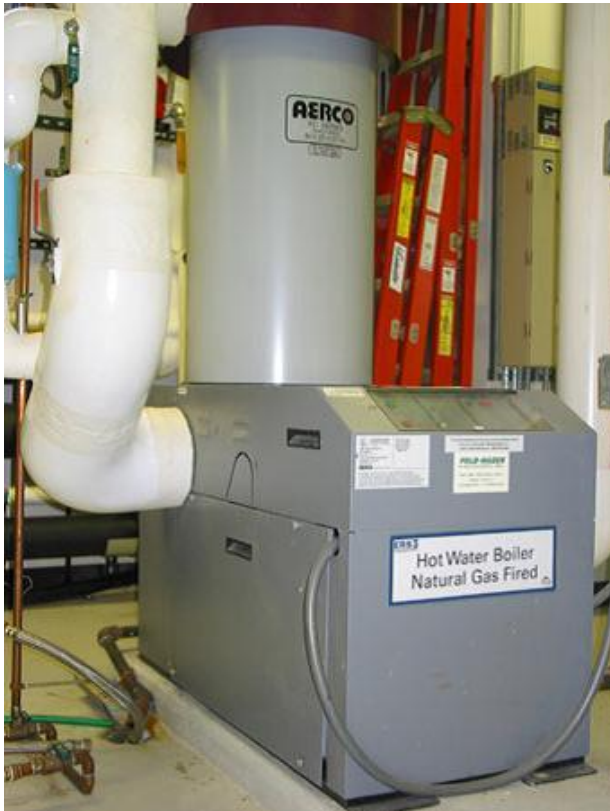
Figure 8: Heating Water Boiler
