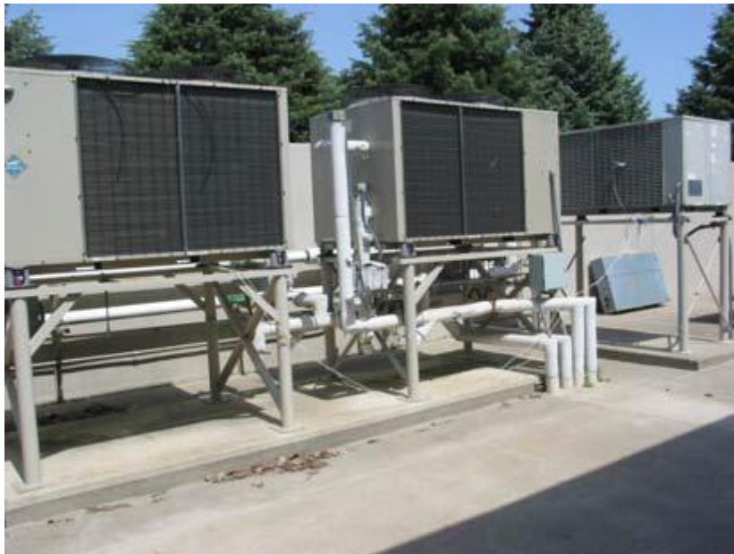
Figure 10: Air Cooled Chillers from left to right ACCH-A, B and ACCH-CH
