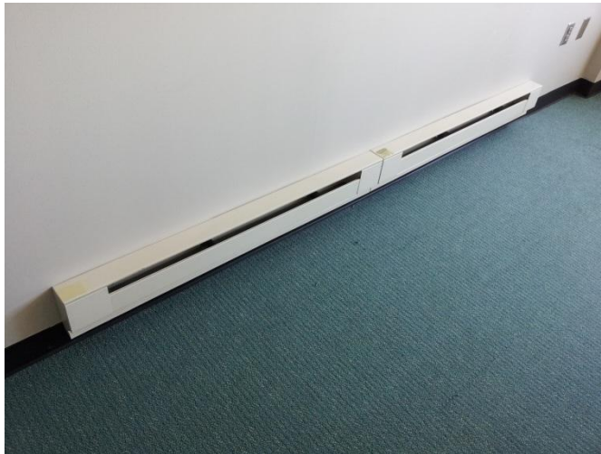
Figure 26: Test Room Baseboard Heaters
