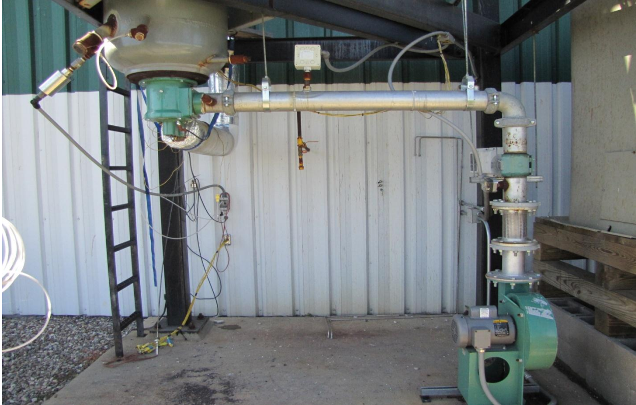
Figure 3.9: Fuel and air inlets, air pump, and thermal gas flow meter.
