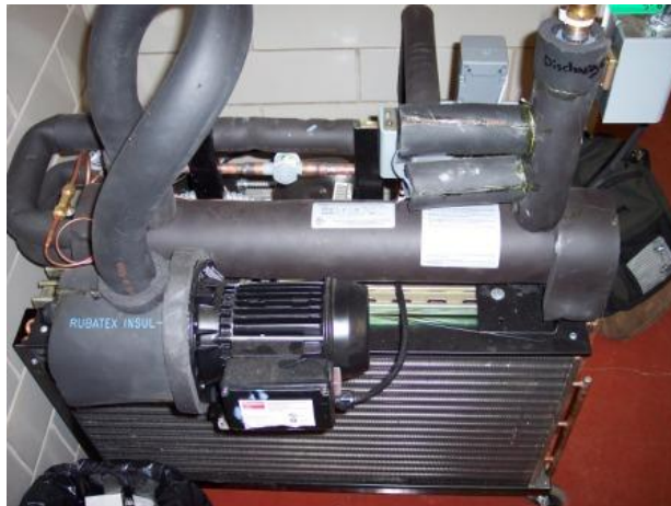
Figure 101. 2.5 ton chiller built from kit
