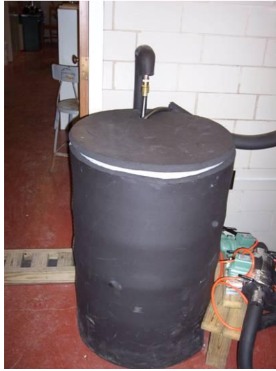
Figure 100. 55 gallon drum for glycol/water thermal storage
