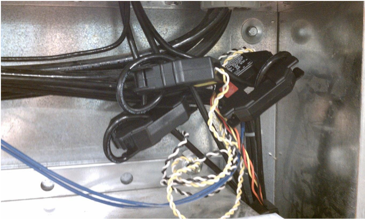
Figure 0.2: Current transducers installed on the return fan power
