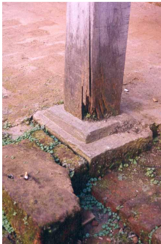
Figure 3.6: Base column rotted due to rain (Nienhuys 2003).
