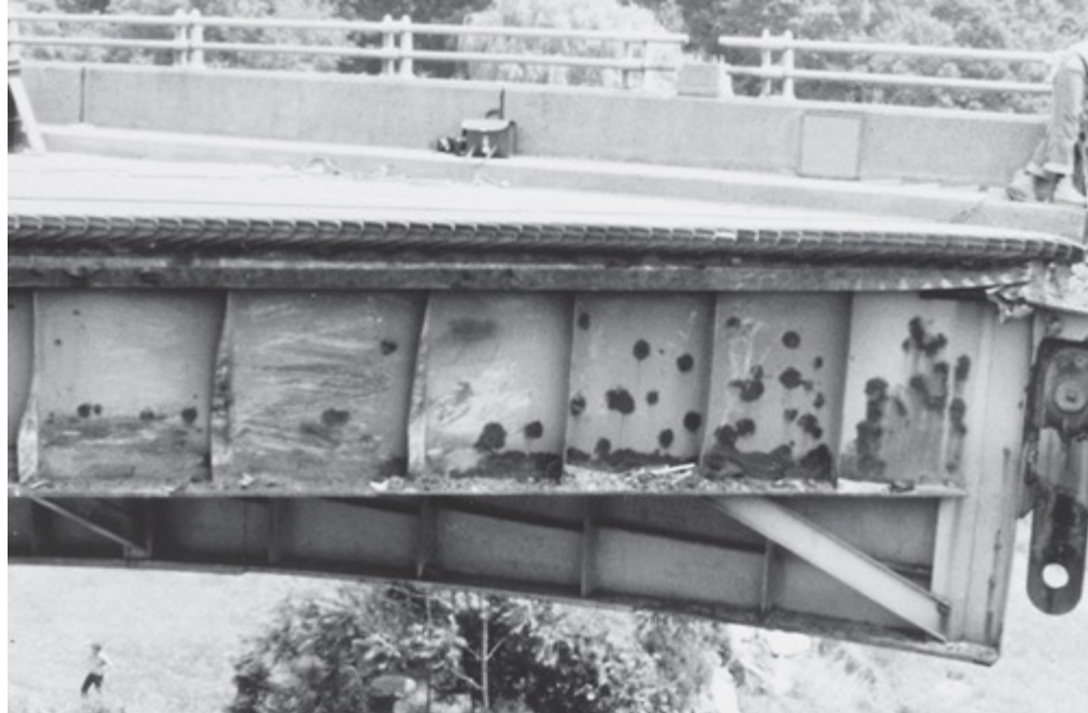
Figure 2.1 Mianus River Bridge collapse (Connor et al. 2005)
