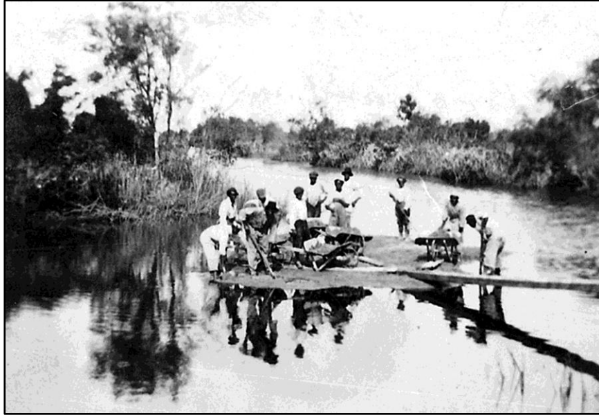
Figure 7.3. Workers repairing a broken rice bank on the Santee Club's Washo Plantation after a hurricane, July 1916. Flood waters had washed much of the bank into the adjacent canal leading from the Santee River, which is in the background of the picture, out of sight. Source: private collection.
