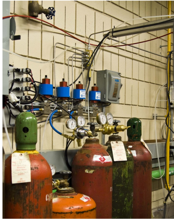
Figure 3.16 - Gaseous cylinders with air actuated valves.
