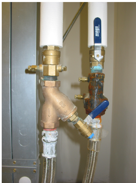
Figure 5.2. Heat pump hook up.
