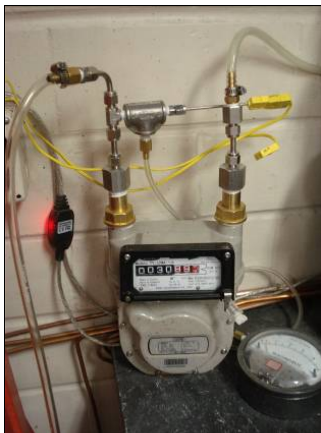
Figure 132. Gas volume meter and pressure gauge
