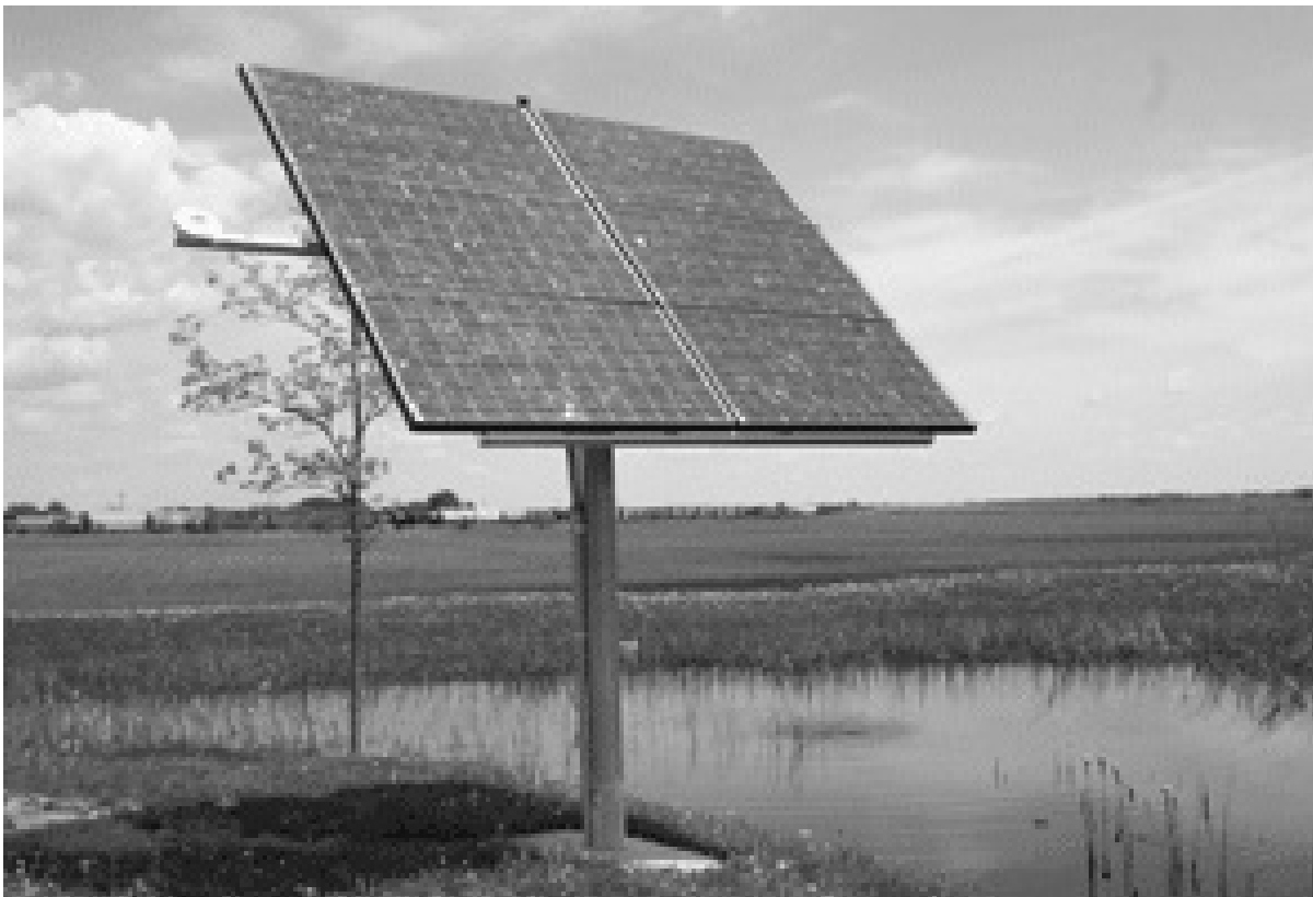
Figure 3.1. Photograph of tracking PV system
