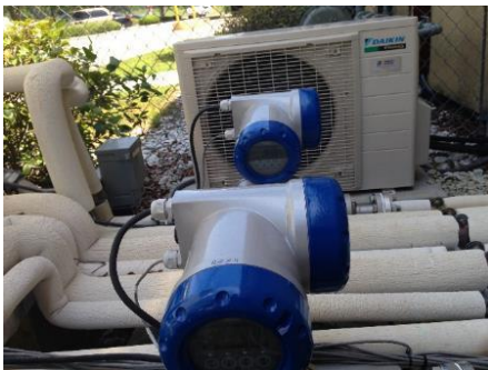
Figure 24. Refrigerant flow meters wired and connected to the DAQ system
