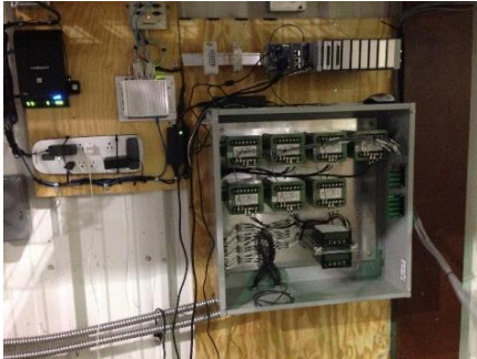
Figure 22. Wattmeters for the AHU's
