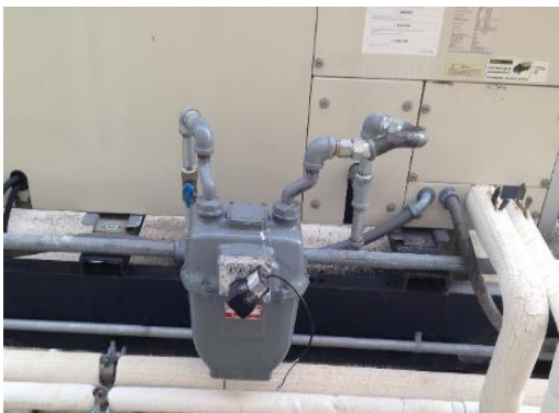
Figure 20. Natural gas consumption meter
