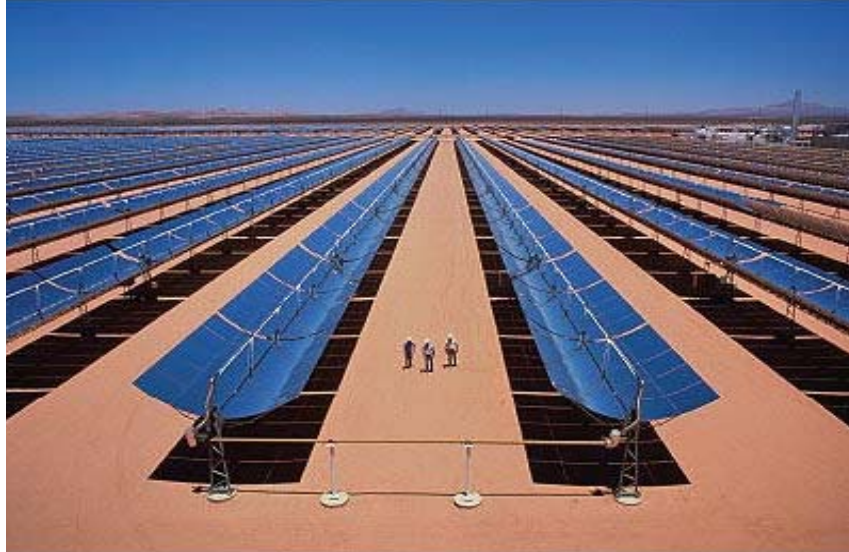
Figure 2.3 Parabolic trough solar collectors [10]
