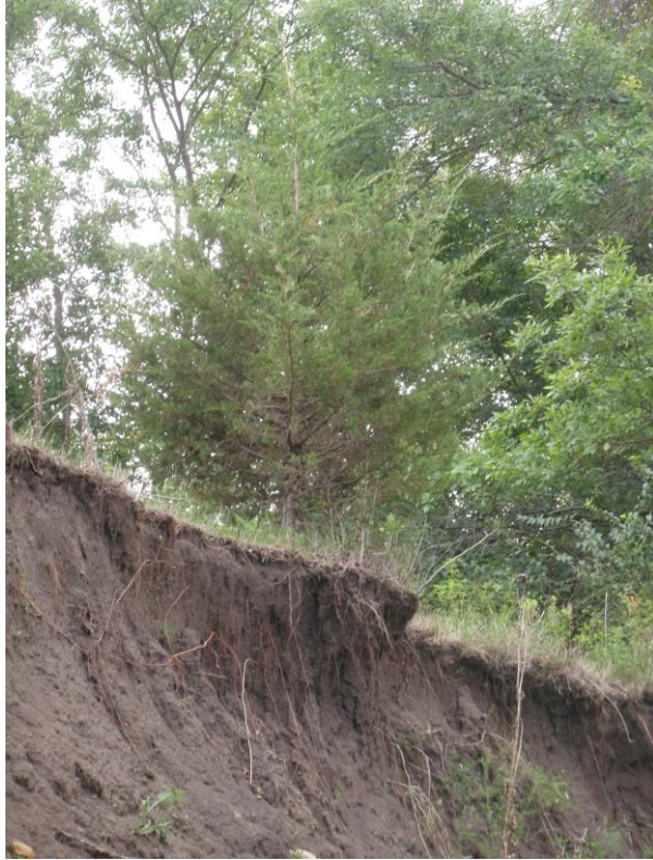
Figure 8: Tree roots stabilizing bank soils. The 10-foot high bank, however, was deeper than the tree's roots. Photo taken August 2012.
