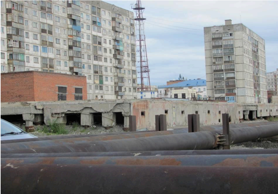
Figure 10. Norilsk City landscape. Aging and neglected Soviet-era housing and industrial utilidors predominate in Norilsk. (Photo: G. Parente)
