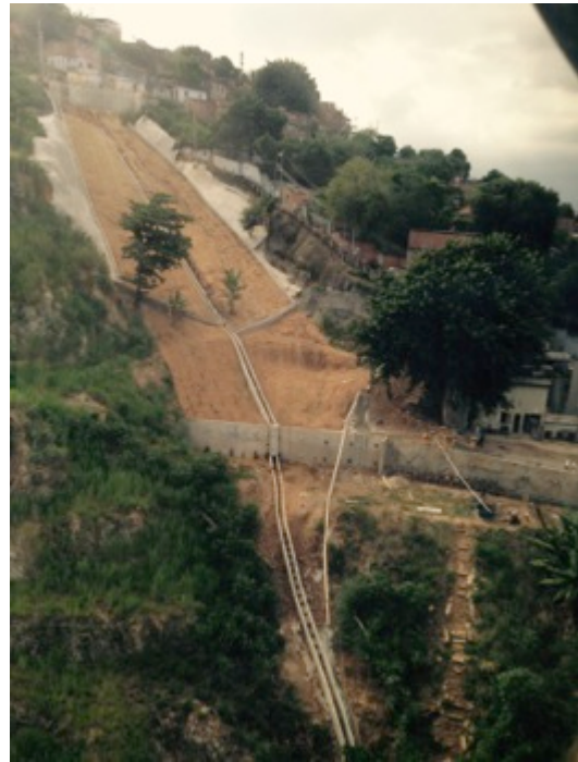
Figure 5.6 New drainage being installed on Adeus. I captured this project being built on a return trip to Complexo in 2015, five years after the construction of the teleferico. Photo taken 24 Mar 2015 by author.
