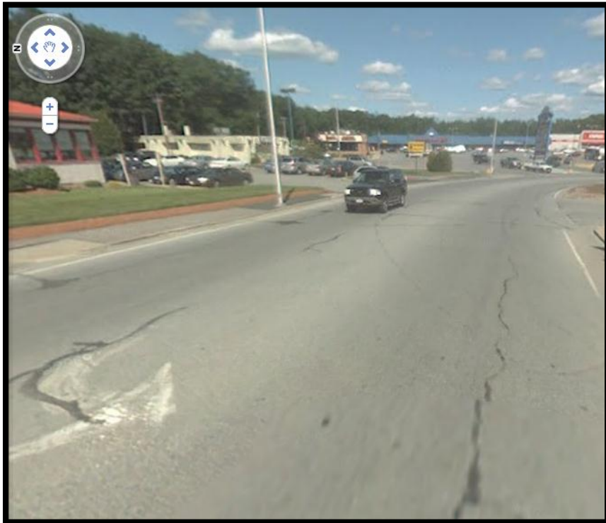
Figure 59. Roadway Segment 155628 Street View – Poor Pavement Markings
