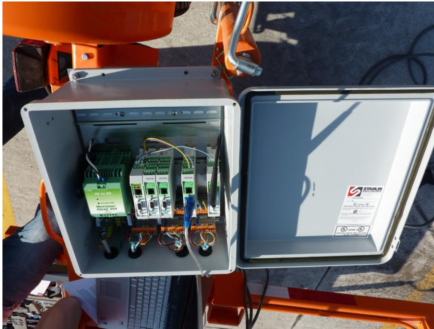
Figure 3.12: Portable sensor pole cabinet
