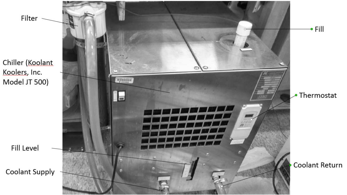
Figure 3.5: Chiller unit with water
