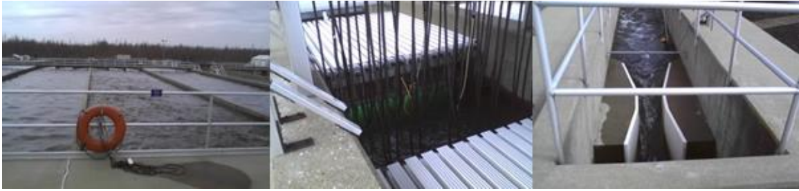
Figure 5.1 Aeration Tank, Ultra Violet Lights, and Point Source
