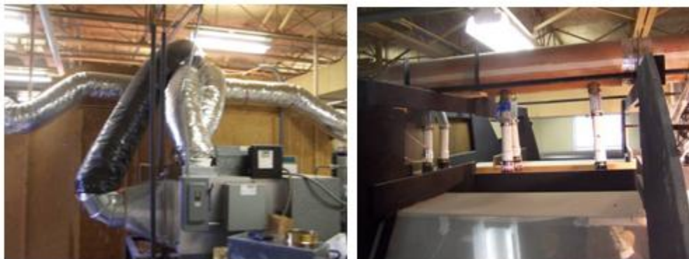
(a) Fan installed behind the cabin (b) Duct and nozzle above the ceiling
