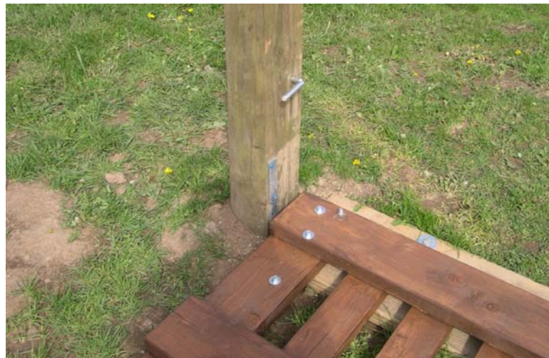
Figure 5.26 Too Ductile To Break Properly When Gate Triggered
