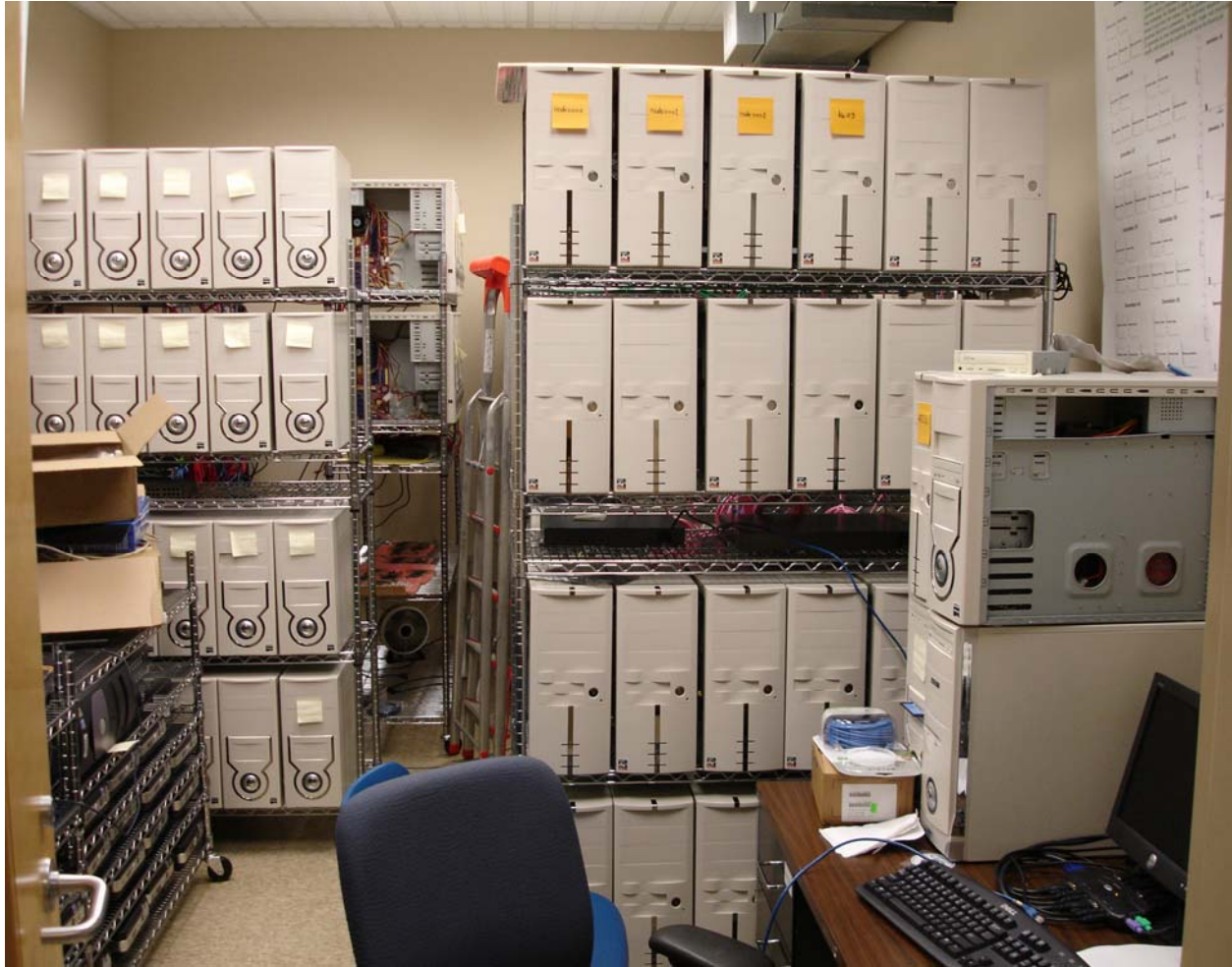
Figure 4-2 Kentucky Fluid Clusters – UK CFD Cluster Room
