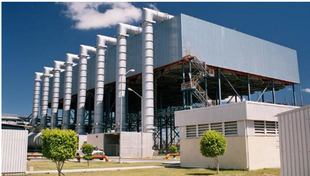
Figure 1.6 Elevated air-cooled condenser array (SPX, 2015)
