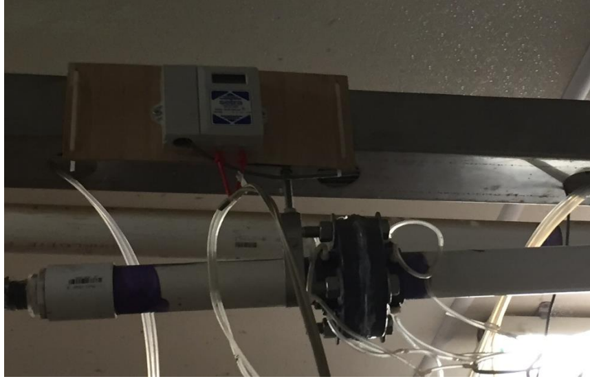
Figure 2.1. The location of a differential pressure transducer in ventilation supply subsystem.
