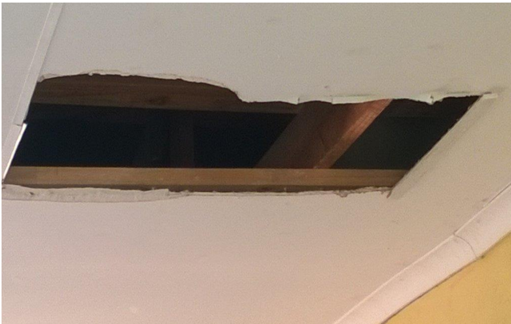
Figure 4.7 Damaged ceiling (vandalism of school property)
