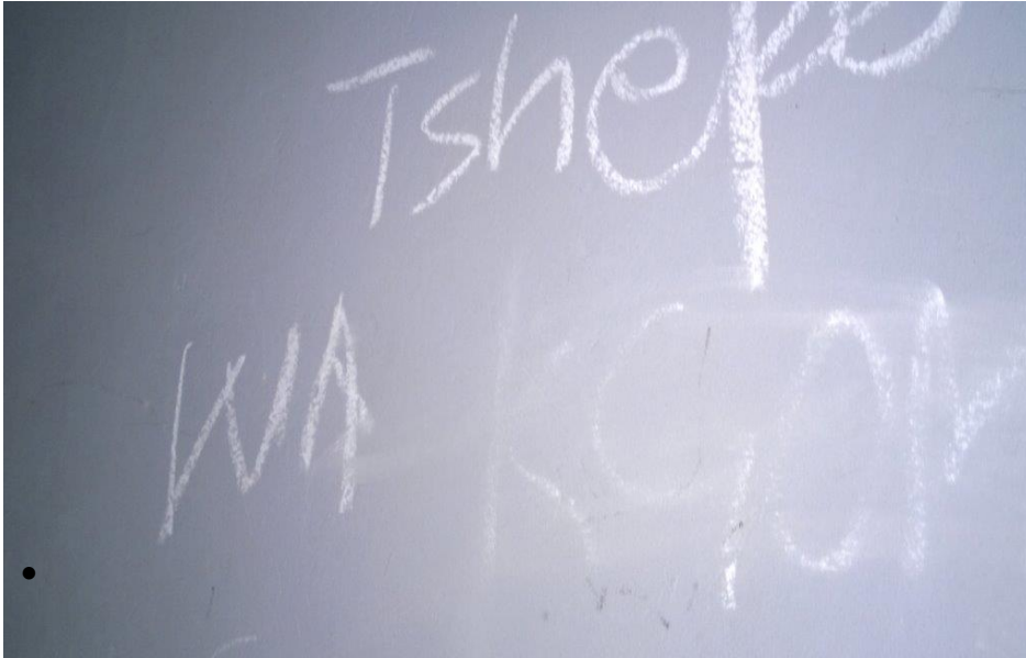
Figure 4.6. Dirtying painted schools walls
