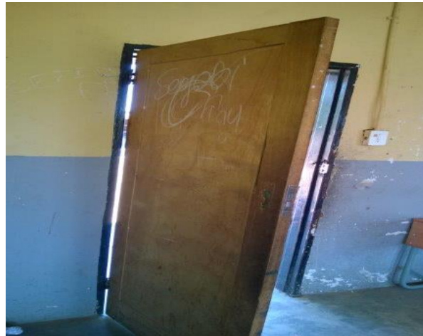
Figure 4.3 Classroom doors cannot be locked owing to vandalism
