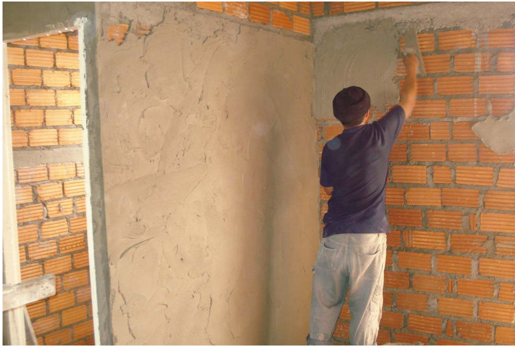
Figure 17: A workman using smooth finishing to cover the brick wall to create a neat appearance
