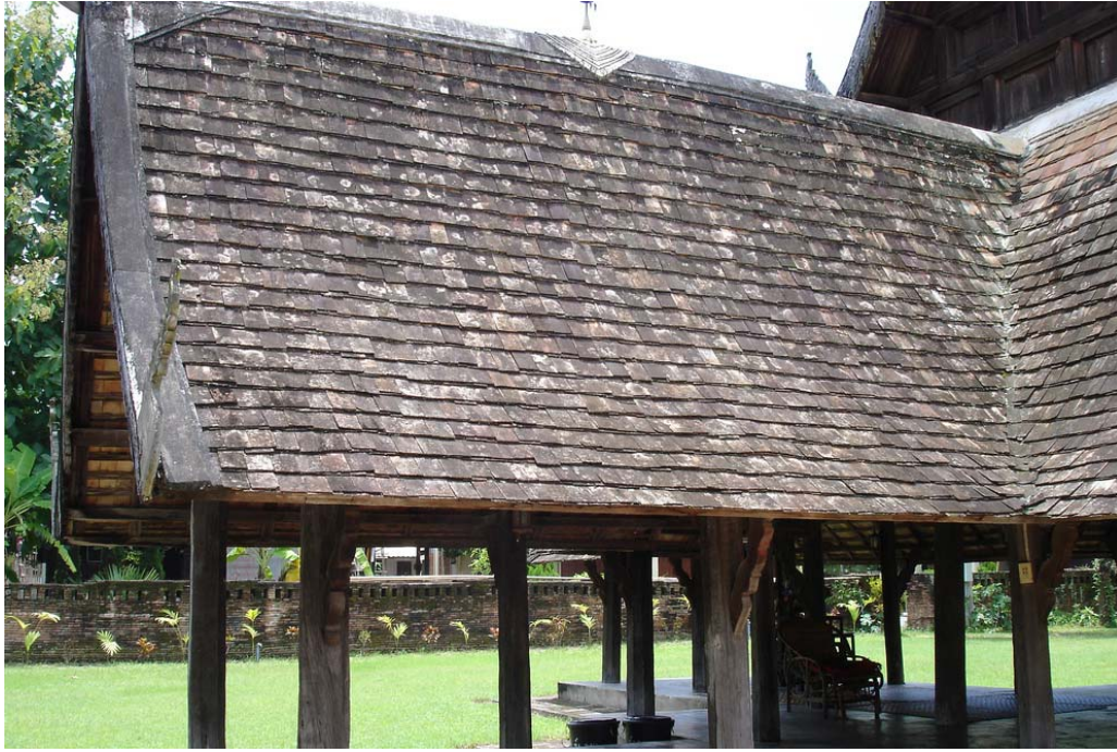
Figure 37: Wood shingle roof tile is very common in the Northern part of Thailand
