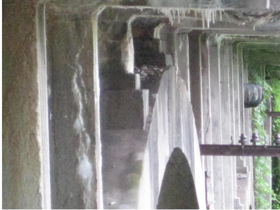
Figure 4.7b –Lack of cracking between the spandrel columns and the arch (photograph taken in June 2009).
