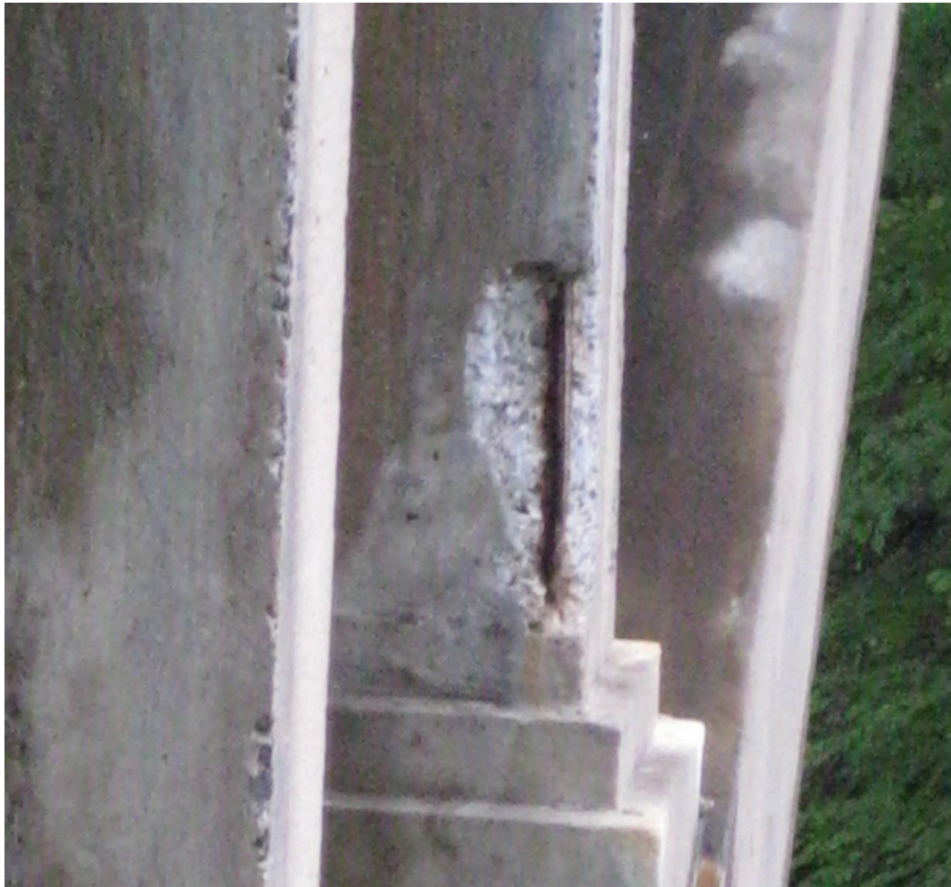
Figure 4.7a – Evidence of reinforcement in the spandrel columns that goes into the arch connection (photograph taken in June 2009).
