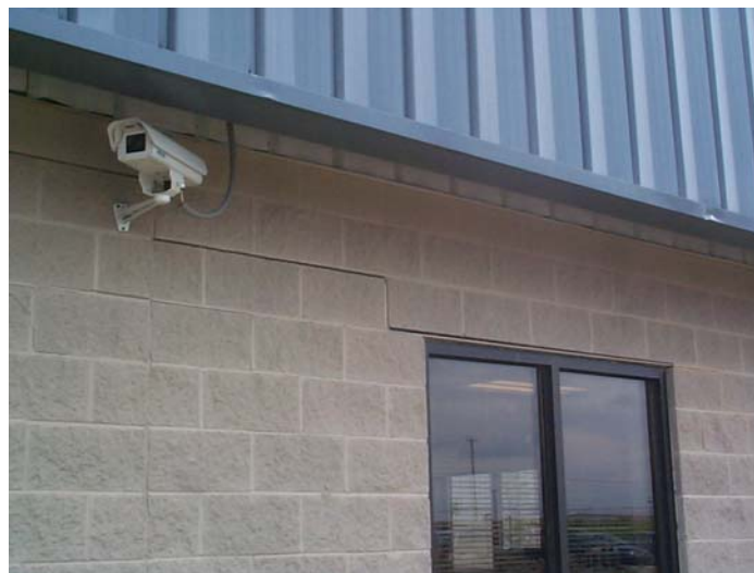
Figure 2.2. Crack in the Coalfields Regional Industrial Park office building (Karem et al., 2007).
