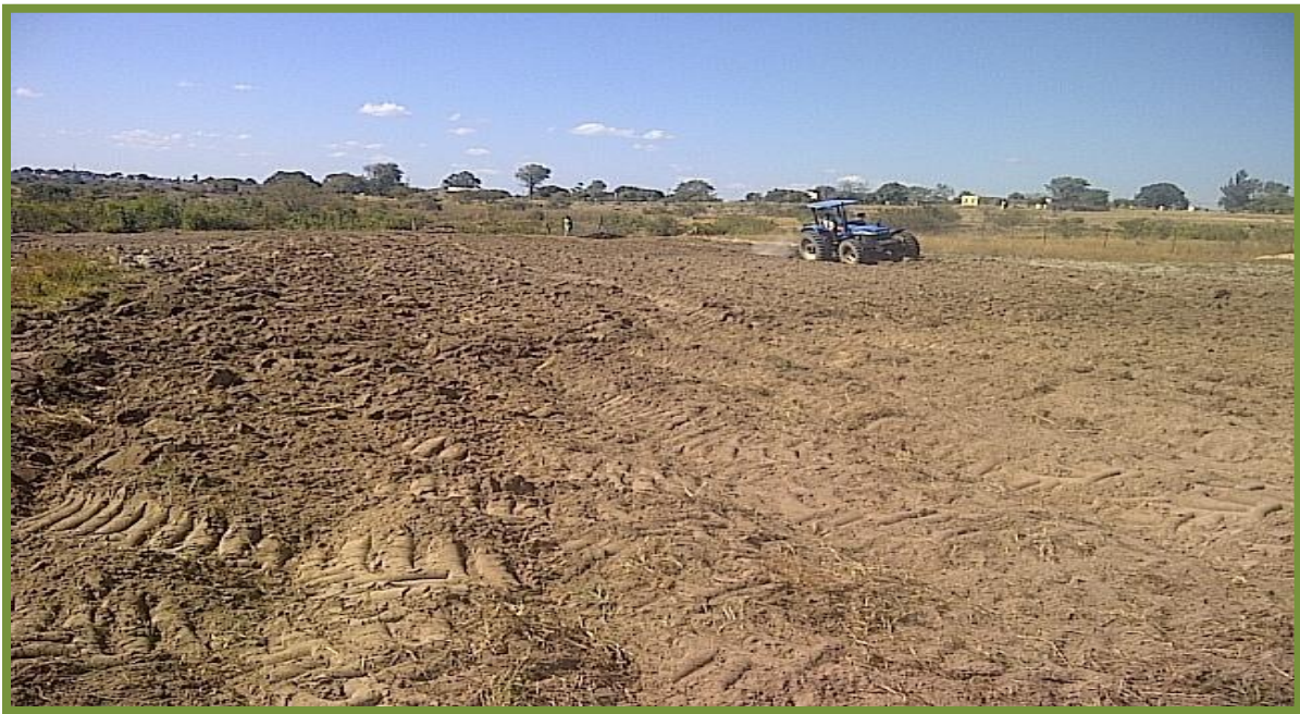
Figure 33: ME tractor at work and the poor performance of the work
