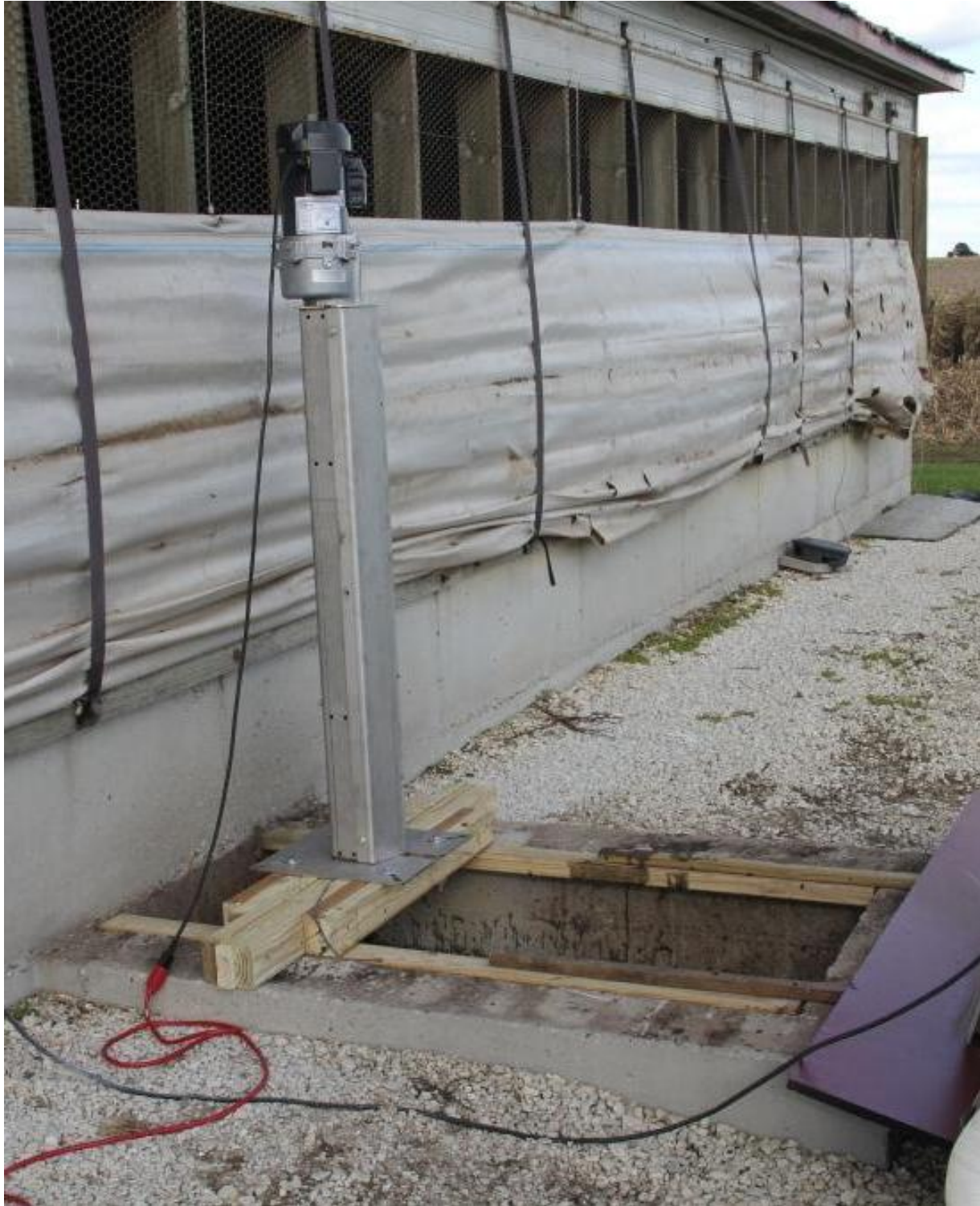
Figure 4.5 - Bracket built to support the mechanical foam mitigation device when installed in the pump-out ports of Barns A and B.
