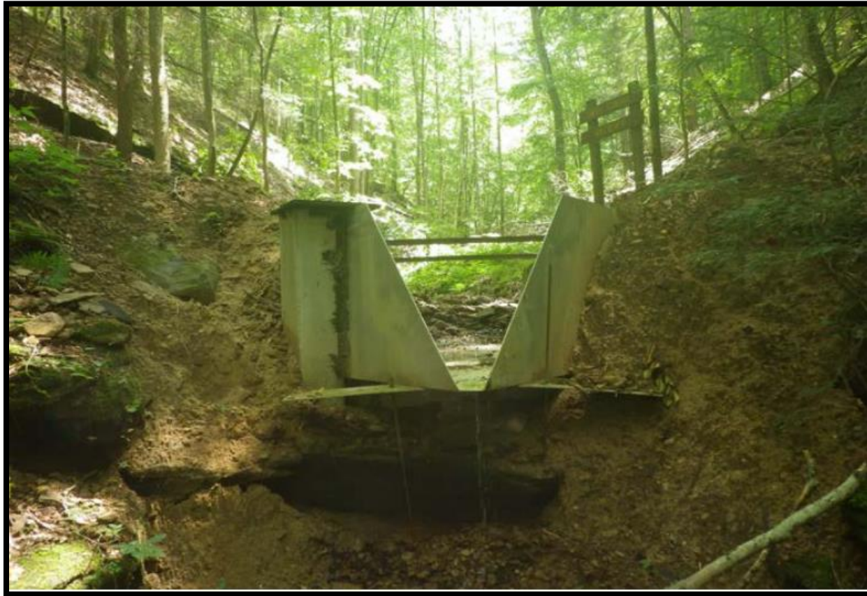
Figure 3.1: Sediment and debris buildup behind WSA flume (2016).
