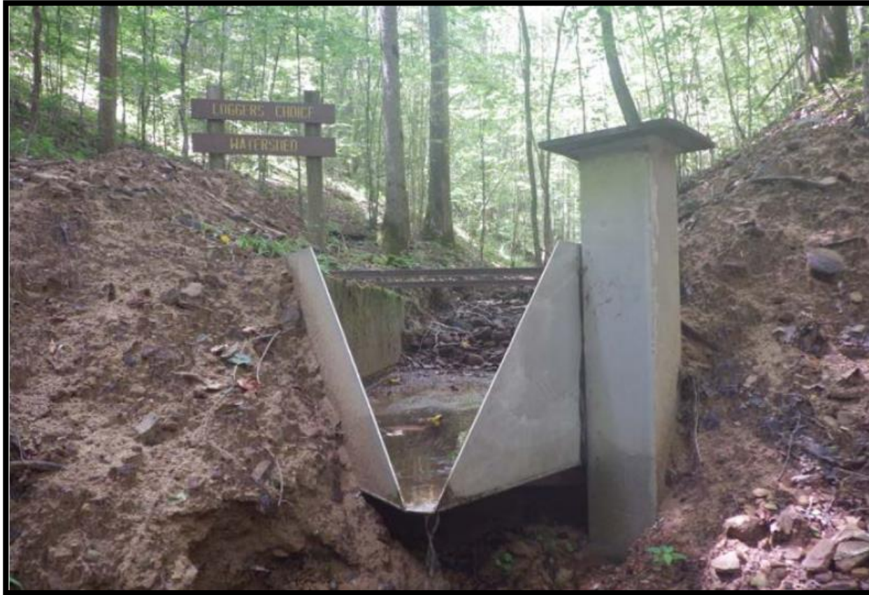
Figure 3.3: Sediment and debris buildup behind WSC flume (2016).
