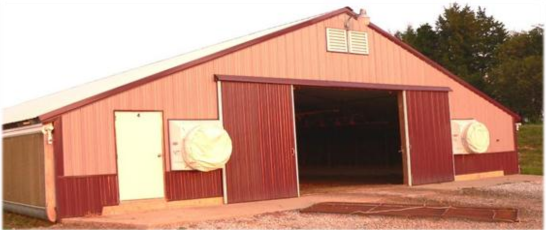
Figure 3.8. West end of Barn 1 at Farm 2. Two 0.91 m diameter Chore Time Fans.
